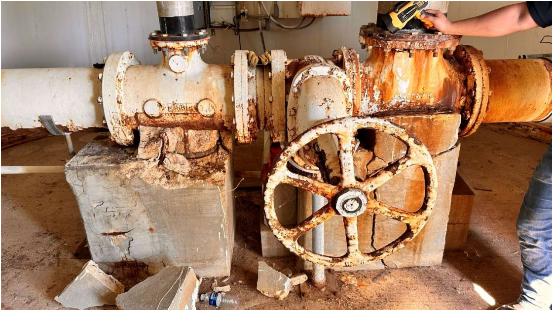
Photo #9: Piping Supports to be removed and replaced.
